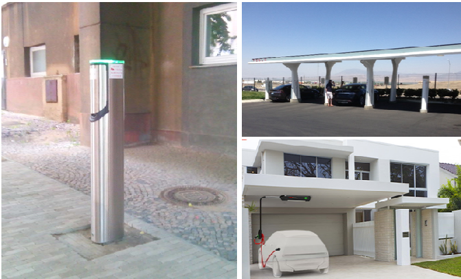
Fig. 6 Examples of EV charging stations: corporate station at Transportation Faculty, CTU in Prague (left), Tesla public charging station with solar energy source (upper right), home charge station by Easycharge (bottom right)
